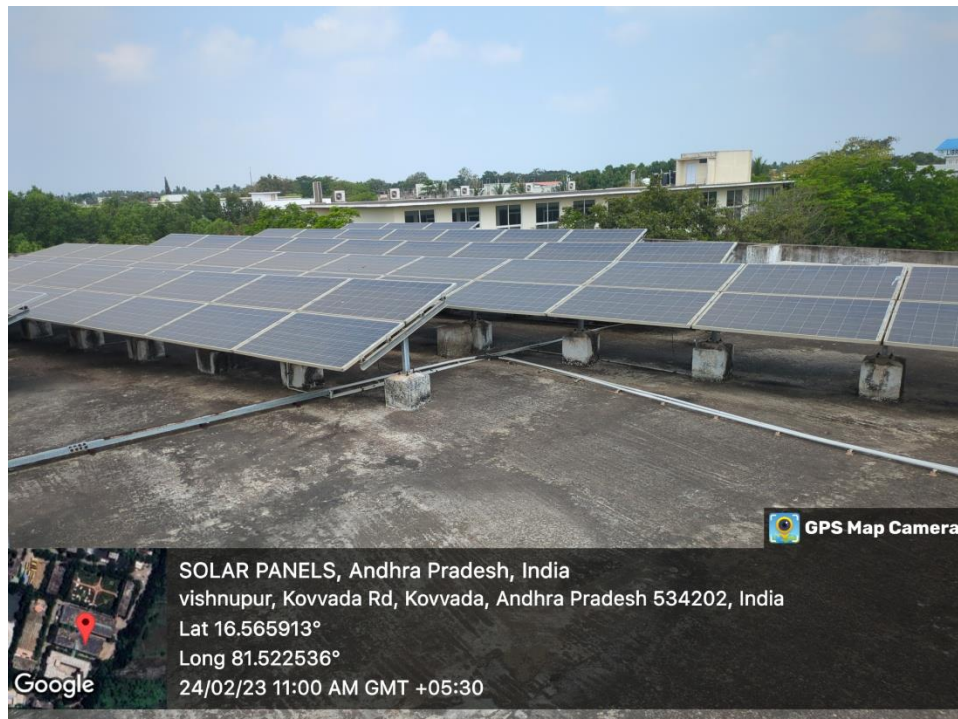
ROOF TOP SOLAR PLANT
